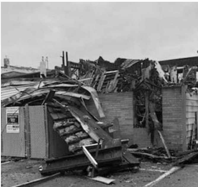
As you can see in all the photos, the building is a loss. But Branch 9 is more than a building.
